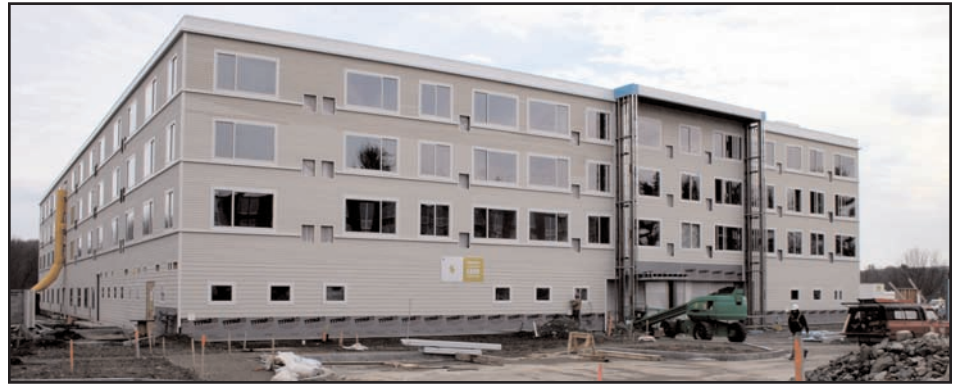
A recent photo of Element, slated to open to the public in early June; not only is this building going to be the first LEED certified hotel in New England, it is on time and under budget as well.
